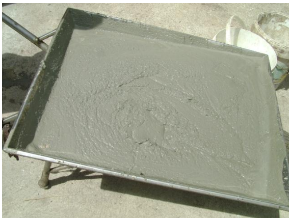
Fig3a. Concrete preparation. A volume of about 50 liters of concrete is required.
