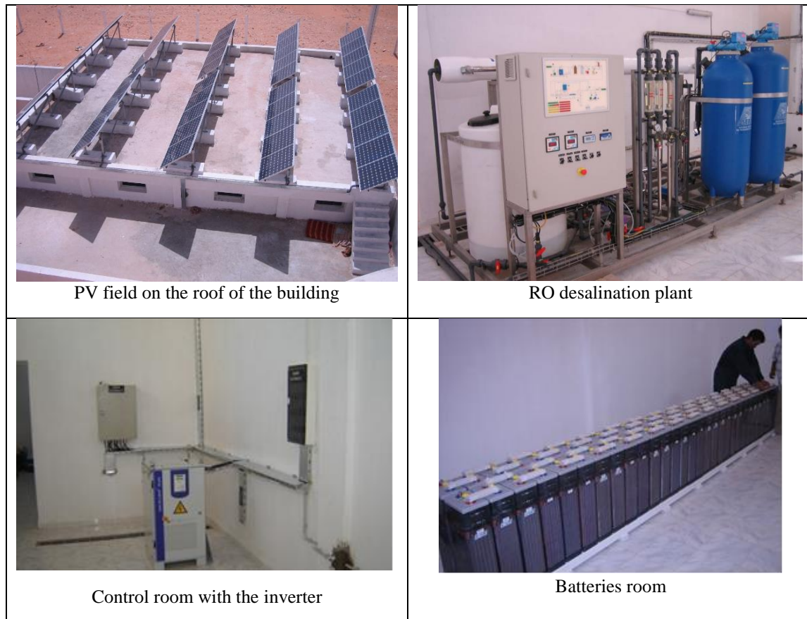
Figure 1. Selection of pictures of the main components of the PVRO system operating in Ksar Ghilène (Tunisia)
